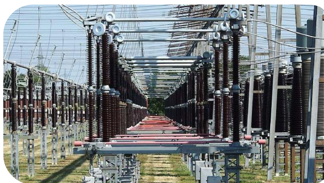
Figure 3.1 Typical AIS external switchgear
