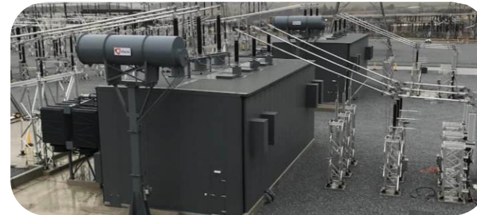
Figure 4.3 A typical transformer acoustic enclosure
